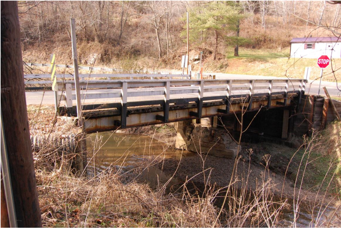
Figure 4: View to the west toward Bridge No. 61 and Little Horse Creek Road
