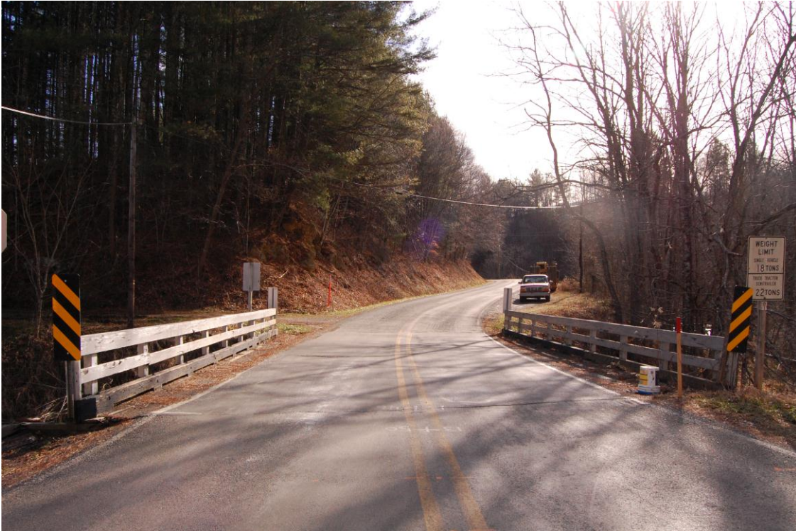
Figure 2: Bridge No. 61 over Little Horse Creek, view to the southwest. Clark-Miller Mill obscured by trees on the right side of photograph
